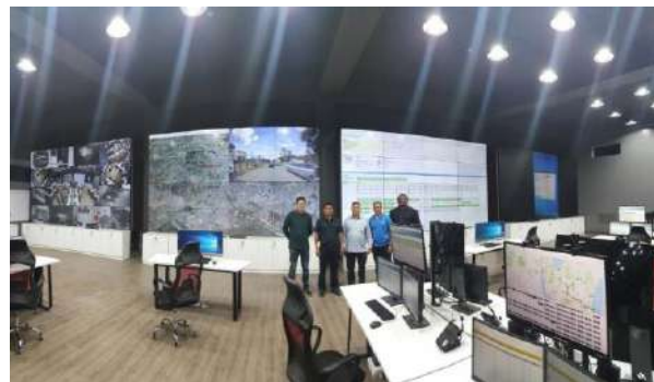
BSMART COMMAND MONITORING CENTRE KENYA, AFRICA
