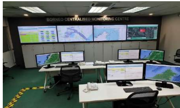
BSMART COMMAND MONITORING CENTRE KOTA KINABALU, SABAH, MALAYSIA
